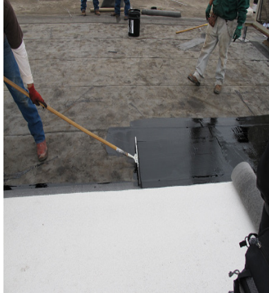
Squeegee apply adhesive for the next course including coverage of the lap of the adjacent sheet
