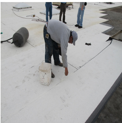
Apply granules to the area Where adhesive has bled-out of the side lap
